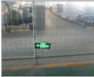
Photo of fire safety equipment Evacuation sign.JPG
