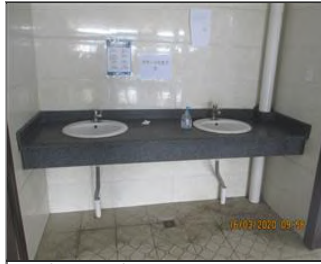
Photo of the sanitary facilities Hand washing facility.JPG
